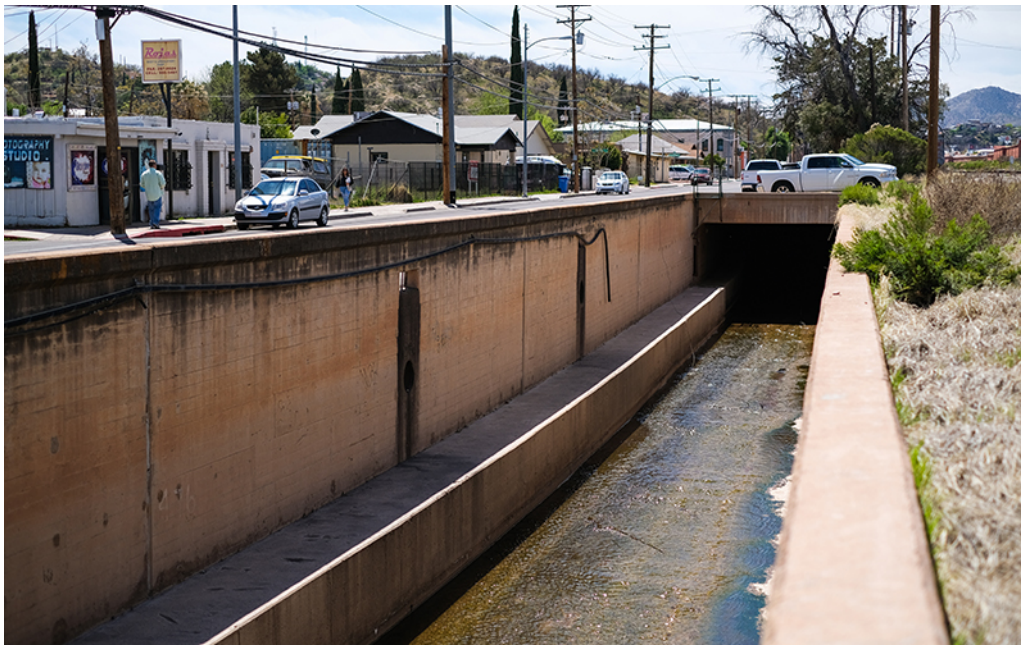
A section of the International Outfall Interceptor is guarded by concrete to protect it from damage, but the majority of the binational sewage pipe runs underground, and depending on the flow of the wash, can be exposed. (Photo by Chloe Jones/ Cronkite News)
